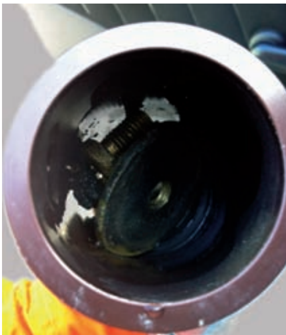
Figure 4: a hydrant that has not been properly maintained.
