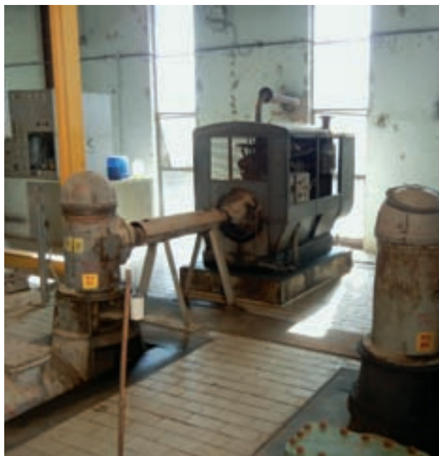
Figure 5: neglected, out-of-service firewater pump.
